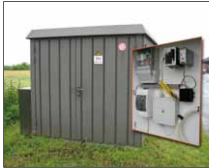
Transformer Station (Example)
